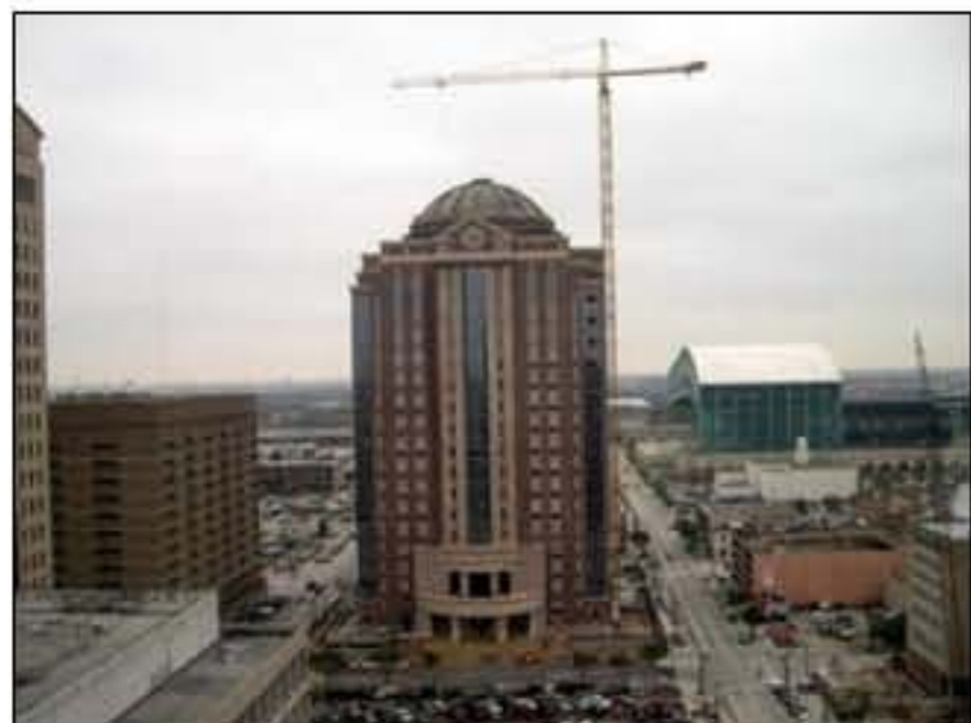
The Harris County Civil Justice Center was under construction when this photo was taken in 2005.
